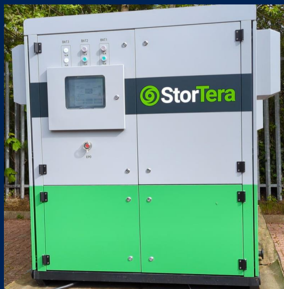
Figure 3: BESS Enclosure Front View
